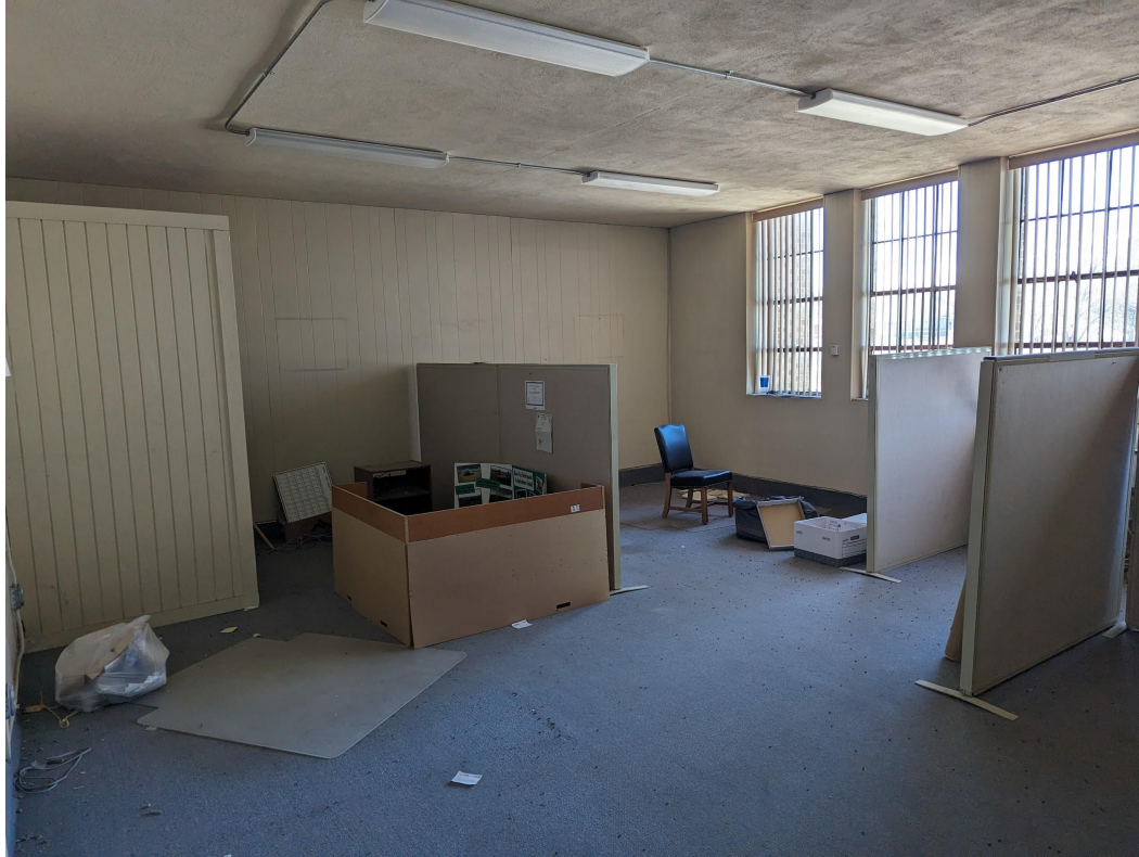
Three rooms are unaffected by leaking but need fresh paint, replacement windows and heating.
