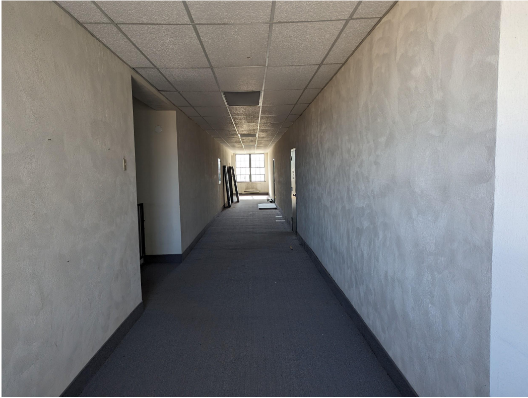
South end of the upper hallway ready for a coat of paint and some carpet.
