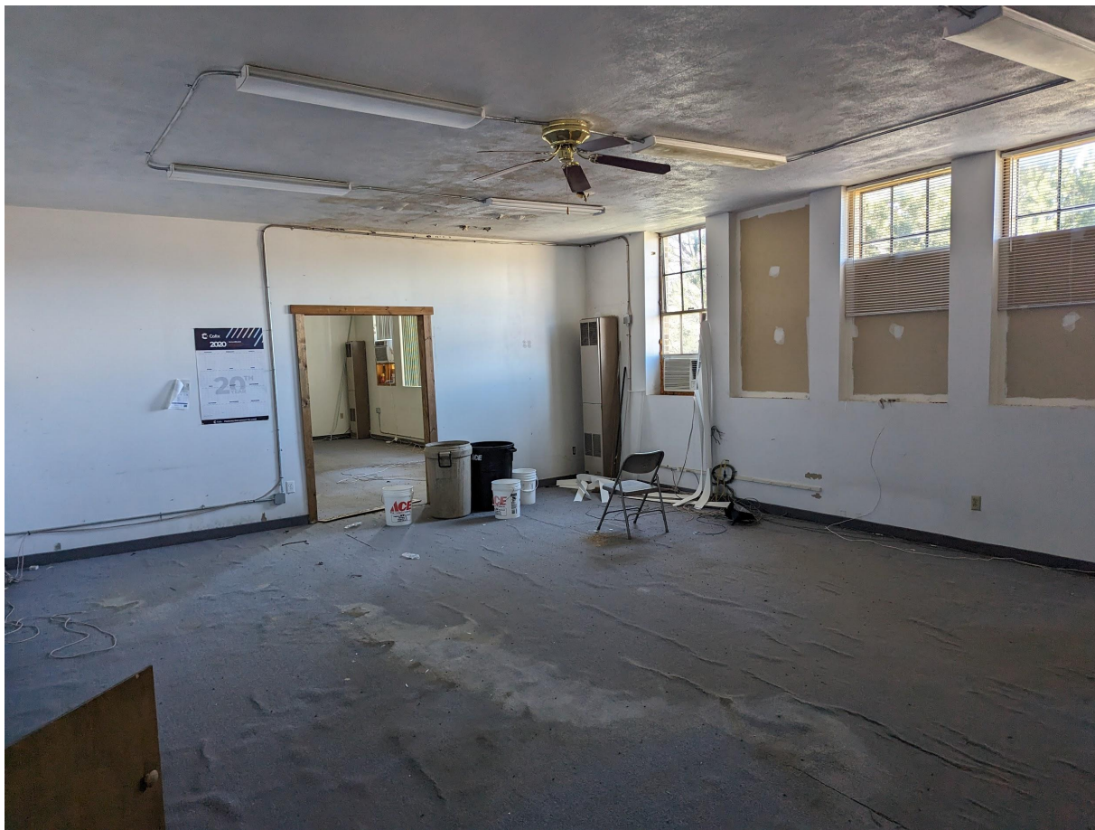
Severe leaking requires ceiling replacement.
